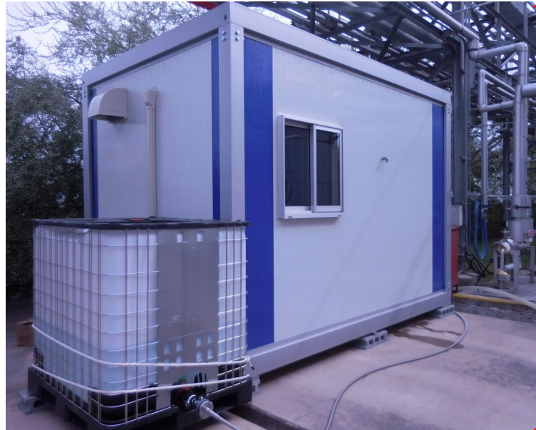
Exterior of electrodialysis test facility
