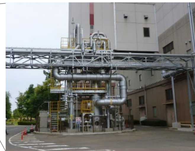
Exhaust gas pretreatment plant (desalination treatment)
