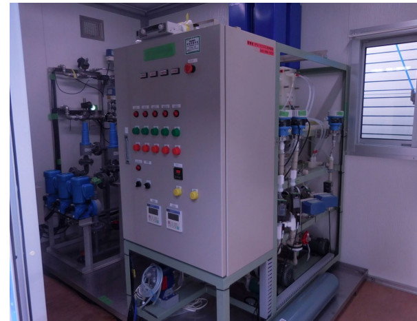
Interior of electrodialysis test facility
